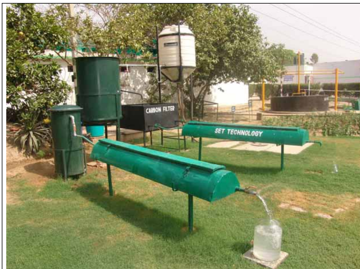
Picture-4 Biogas plant effluent treatment system
