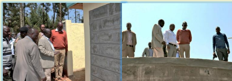
Left: WSTF CEO, Ismail Shaiye and H.E Joshua Irungu viewing the newly built Sanitation Facilities at Kite Secondary School. Right: Viewing of the 135m 3 Masonry Water Tank under the WSTF Joint 6 Program
