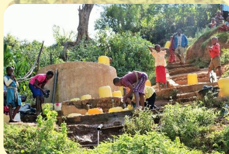
Rehabilitated and Protected Kaithamba Springs by Bwathonaro Water Resources Users Association (WRUA) in Meru County
