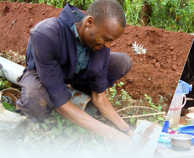
Murang'a Water & Sanitation Staff laying water pipes for Muchungucha Water Supply Project
