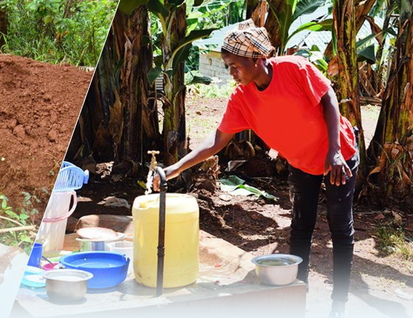
A domestic water consumer drawing water from a newly installed water connection by Muranga Water & Sanitation Company in low income areas
