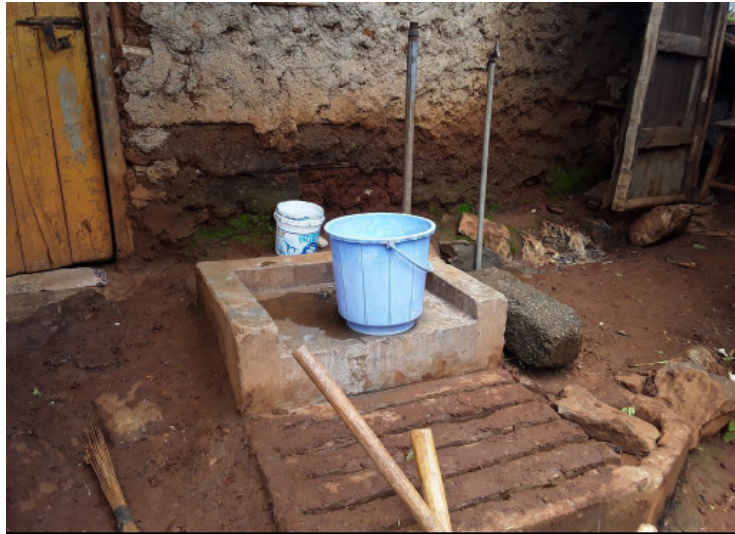
Yard tap, Langas And Kingongo Water Kiosks Rehabilitation, UPC (2012/13), Uasin Gishu County
