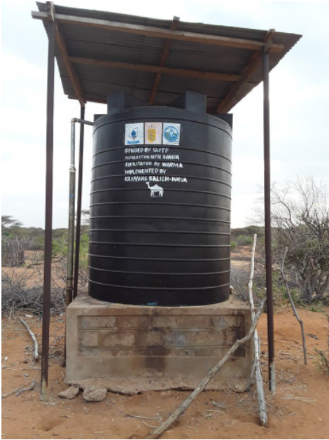
Rainwater harvesting tank, Kanyang Balich, MTAP I (2015/16), Garissa County
