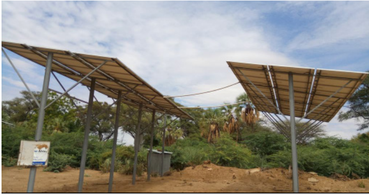
Solar pumping system, Kanamkemer Solar Water Project, UPC Programme (2016/17), Turkana County
