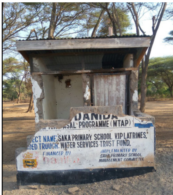
Non-operational VIP Latrine, Saka Primary School, MTAP I (2013/14), Garissa County
