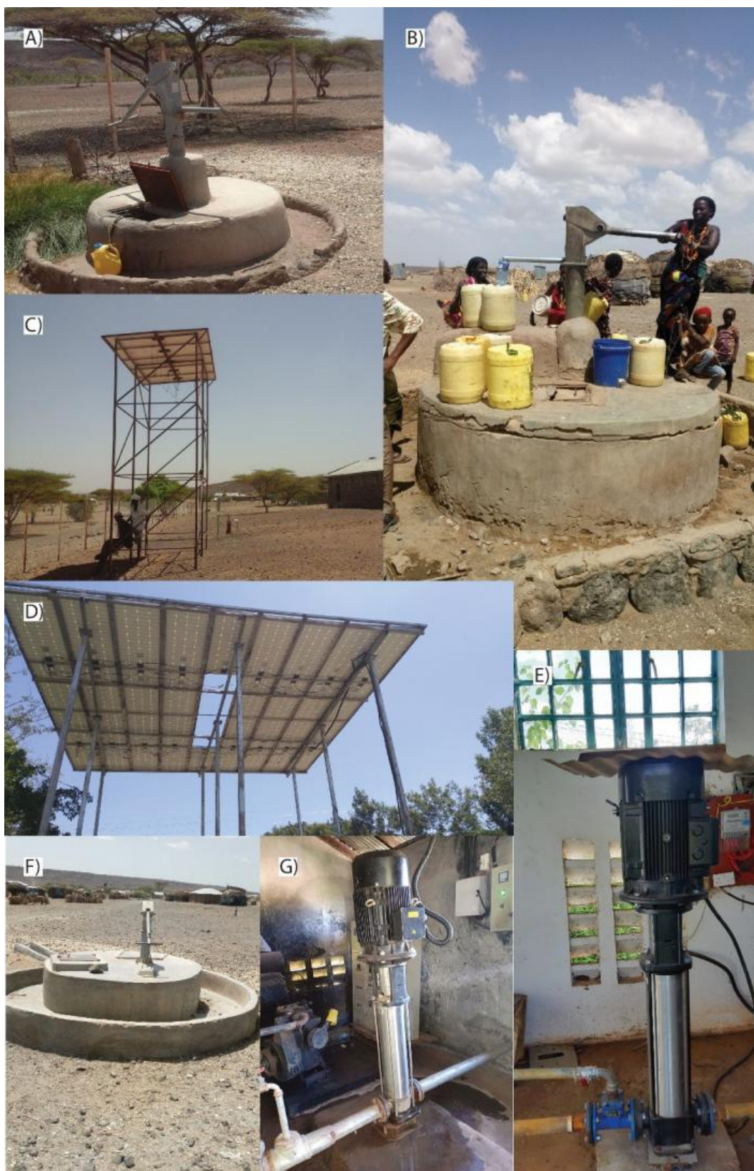
Figure 93. Pumps and Energy sources. A)-C) Hand pumps and solar panels, Galasa Water project, MTAP I FY 2014/15, Marsabit county; D) Solar panels, Nyakona Water Users Association project, J6P FY 2017/18, Migori county; E) Electric pump, Uriri/Bware Water & Sanitation Project, J6P FY 2017/18, Migori county; F) Non-operational hand pump, Galasa Water project, MTAP I FY 2014/15, Marsabit county; G) Electric pump, Kimng'oror Water Users association, J6P FY 2017/18, Nandi county.
