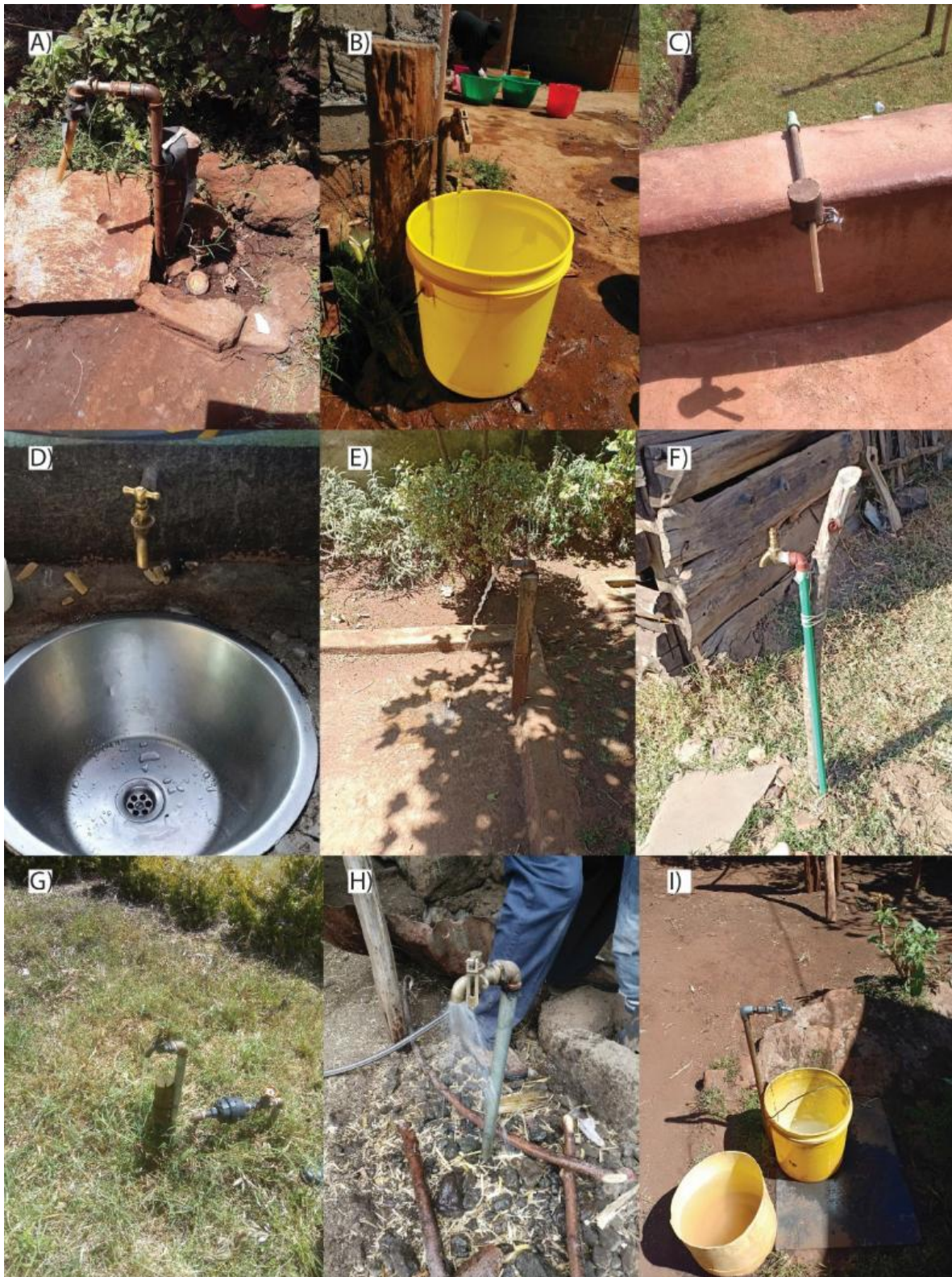
Figure 91. Individual connections. A) Indian Burzar Water Project, UPC FY 2014/15, Kiambu county; B) Mairo Inya Water Project, UPC FY 2016/17, Nyandarua county; C) Nyagacho, Satellite & Chebocho Water Project, UPC FY 2016/17, Kericho county; D) Iten Keriobangi Water Project, UPC FY 2013/14, Elgeiyo Marakwet county; E) Kapngetuny Showground Water Project, UPC 2013/14, Nandi county; F) Cheptil dam Water Users association, J6P FY 2017/18, Nandi county; G) Katheri Nyariginu water project, J6P FY 2017/18, Laikipia county; H) Kiwanja Ndege/Industrial Area Water Project, UPC FY 2016/17, Nakuru county; I) Kapngetuny Showground Water Project, UPC 2013/14, Nandi county.
