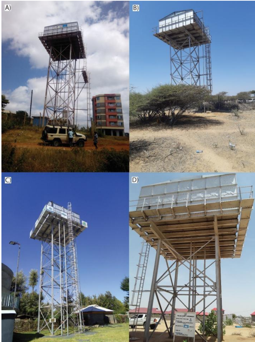
Figure 86. Sectional steel tanks. A) Indian Burzar Water Project, UPC FY 2014/15, Kiambu county; B) Boji Garas Community water & sanitation project, MTAPII FY 2016/17, Wajir county; C) Katheri Nyariginu water project, J6P FY 2017/18, Laikipia county; D) Kanamkemer Solar Water Project, UPC FY 2016/17, Turkana county.
