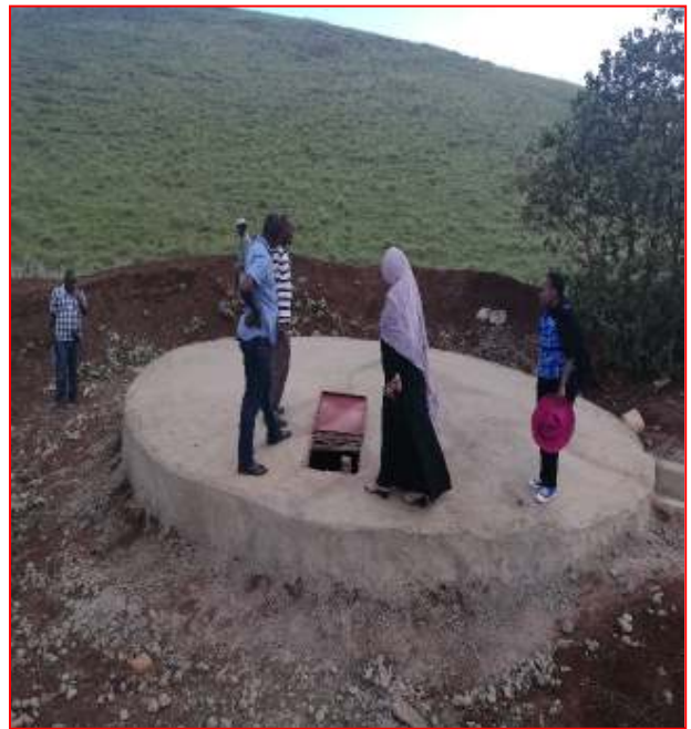
Underground Water tank – Badha Hurri WRUA
