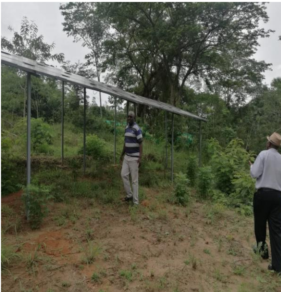
Solar energy panels installed by Majimboni Water Project to supplement the diesel pumps
