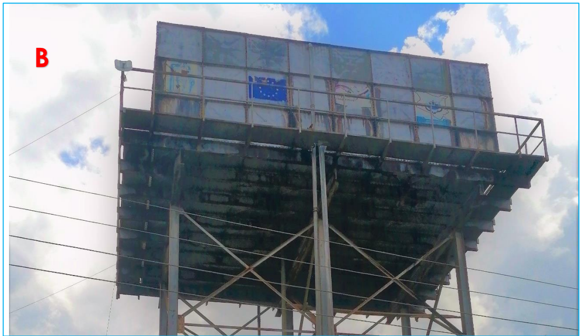
Figure 76: Elevated steel tanks.
