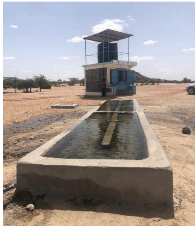
A filled animal watering trough at Lokichar Water Project, Turkana County
