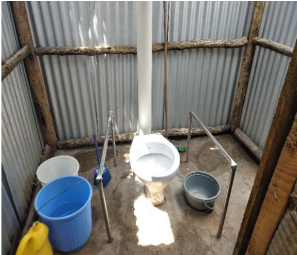
Interior of a PLWD-friendly latrine in Kakuma with a sit and support bars
