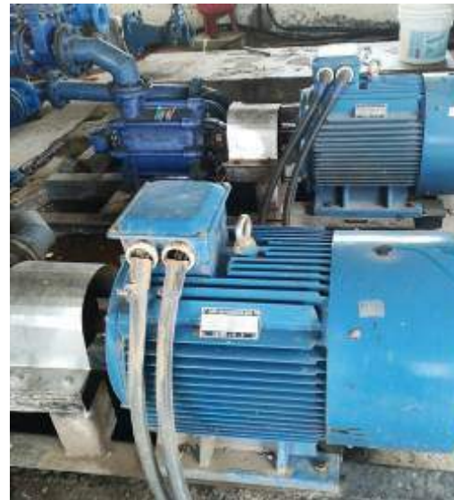
Electric pump in Naivasha water project in Nakuru County
