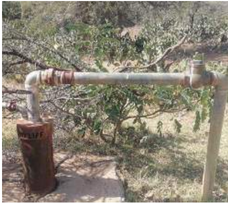
Doldol Water Project in Laikipia
