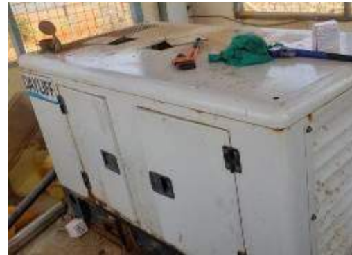
Diesel Pump in Shimbrey water project in Garissa
