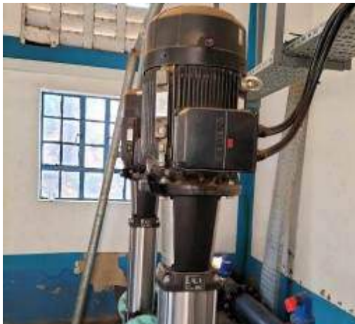
Electricity mains in Kisumu water extension subproject in Kisumu
