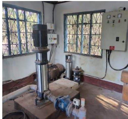
Hybrid Pump in Majimboni Muungano Water Project in Kwale
