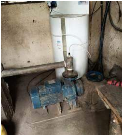
Electric pump in Kinna water project in Isiolo
