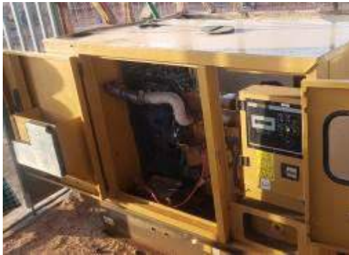
Diesel Pump in Shebta-aad Water Project in Garissa
