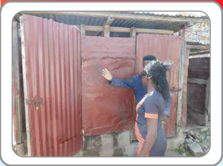
TOILET "A" BEFORE REHABILITATION
