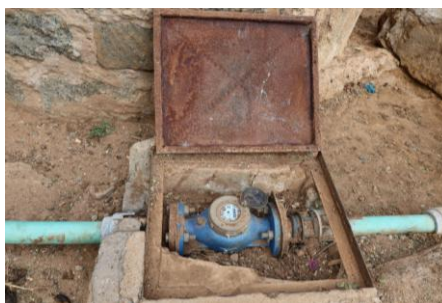
Flanged bulk water meter connection in Machakos County
