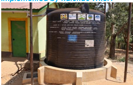
10m 3 Rainwater harvesting tank at Mutula Primary School implemented by Upper Thua WRUA
