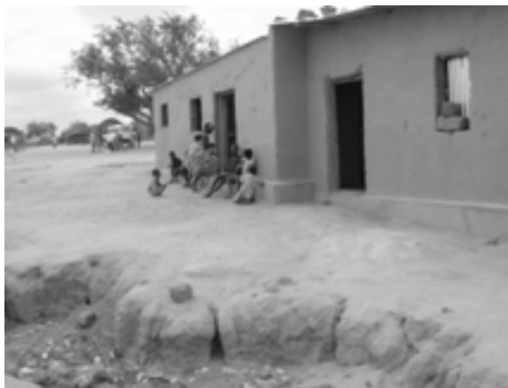
A new health post at an internally displaced persons (IDP) camp – Pomba Nova – near Sumbe Angola. The Health post has no water supply.
